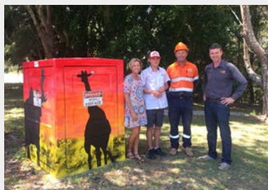
Essential Energy's partnership with House With No Steps helps reduce the incidence of graffiti on Essential Energy assets.
