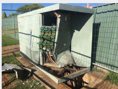
Essential Energy's network is impacted by motor vehicles accidents, such as the damage caused to this padmount substation in Dubbo.
