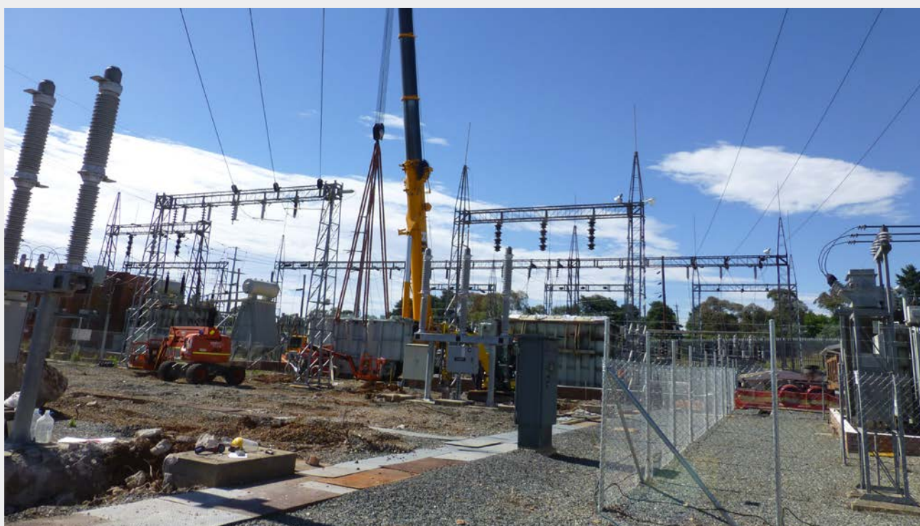
Essential Energy undertaking work for the Cooma zone substation augmentation – installing the 20MVA 66/11kV transformer.
