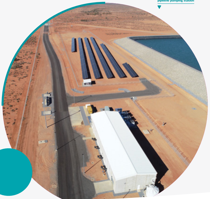
Murray River to Broken Hill pipeline pumping station
