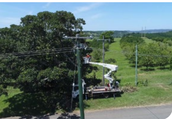
Vegetation management is critical for maintaining network reliability and resilience and reducing network safety risks.
