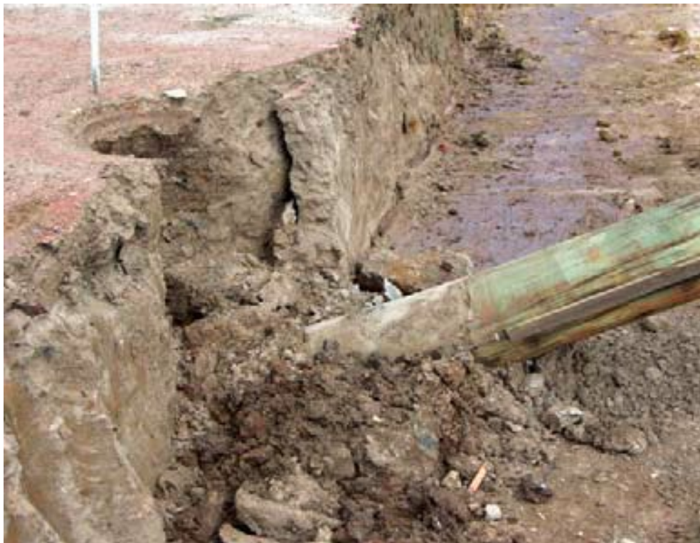
Excavation causing pole collapse.
