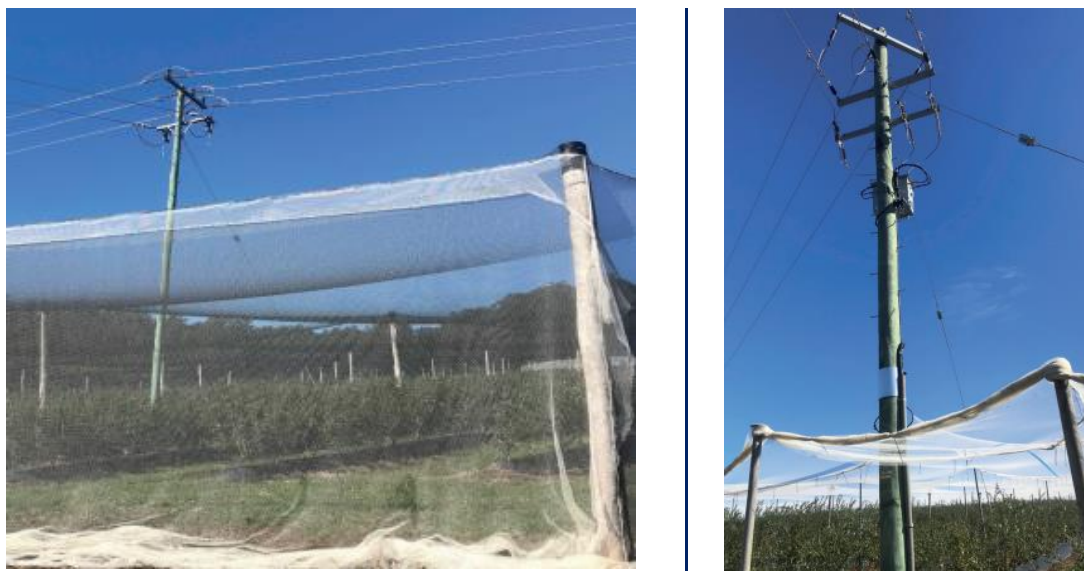
Figure 19: An example of netting and catenaries which are illegally encroaching on the power pole and powerlines
