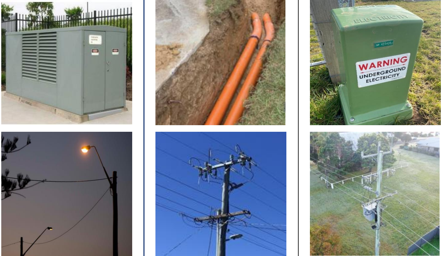
Figure 2: Essential Energy electrical network assets
