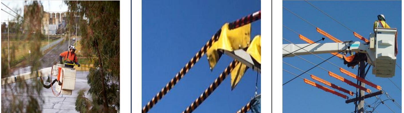
Figure 12: working near overhead powerlines
